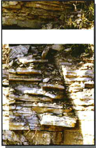
Fractured limestone bedrock presents risk of groundwater contamination.
