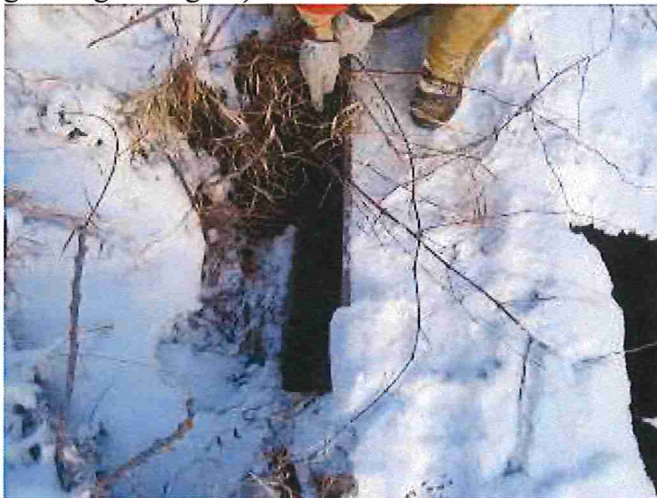
void behind headwall, approx. 2-3' deep.
